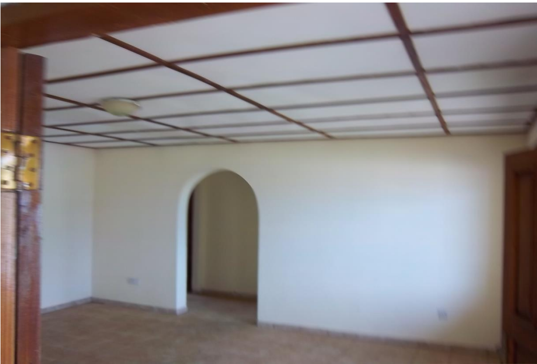
Internal view showing the lounge and entrance arch way to the bedrooms
