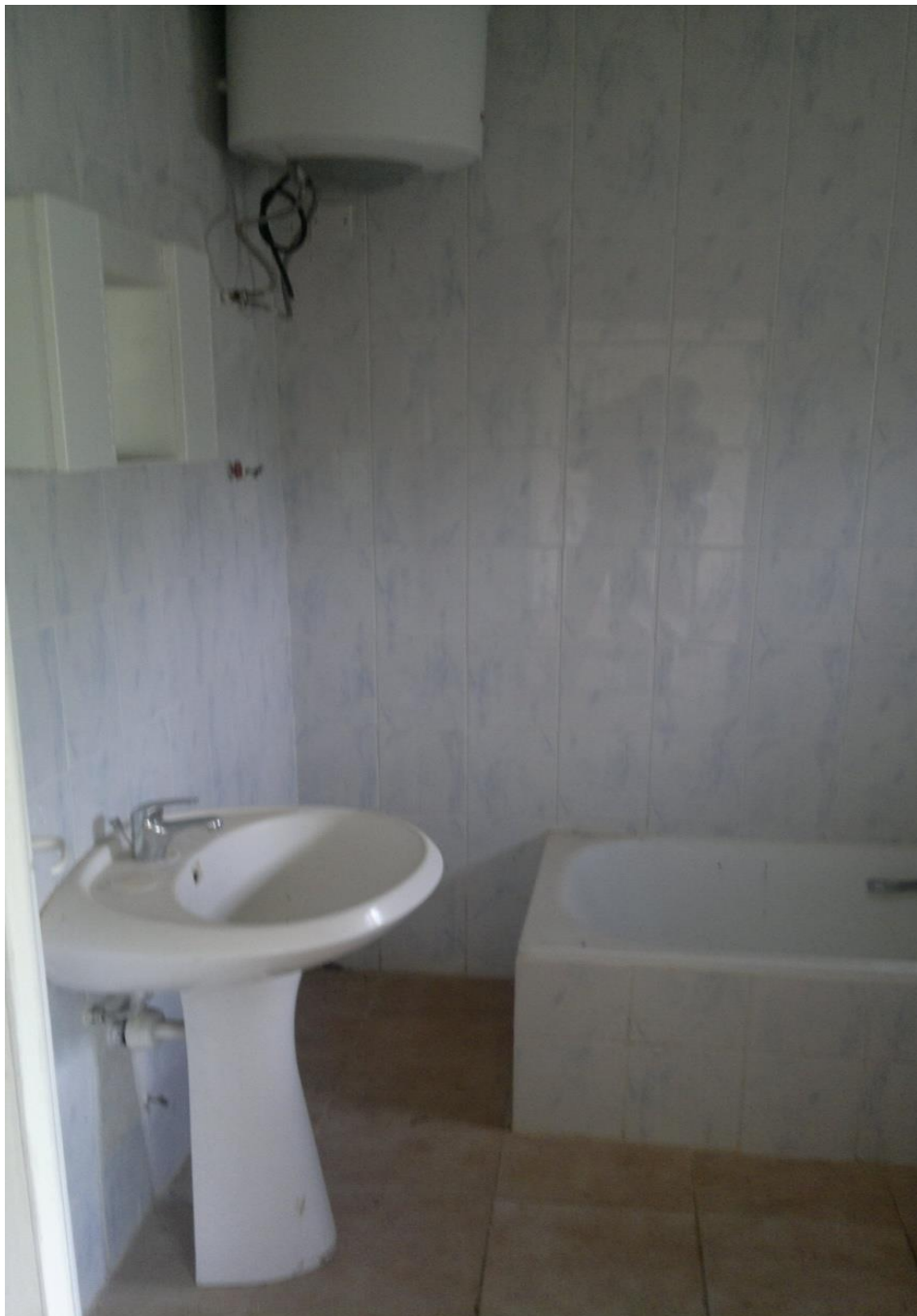
View showing the wash hand basin, water heater and bath tub in the toilet
